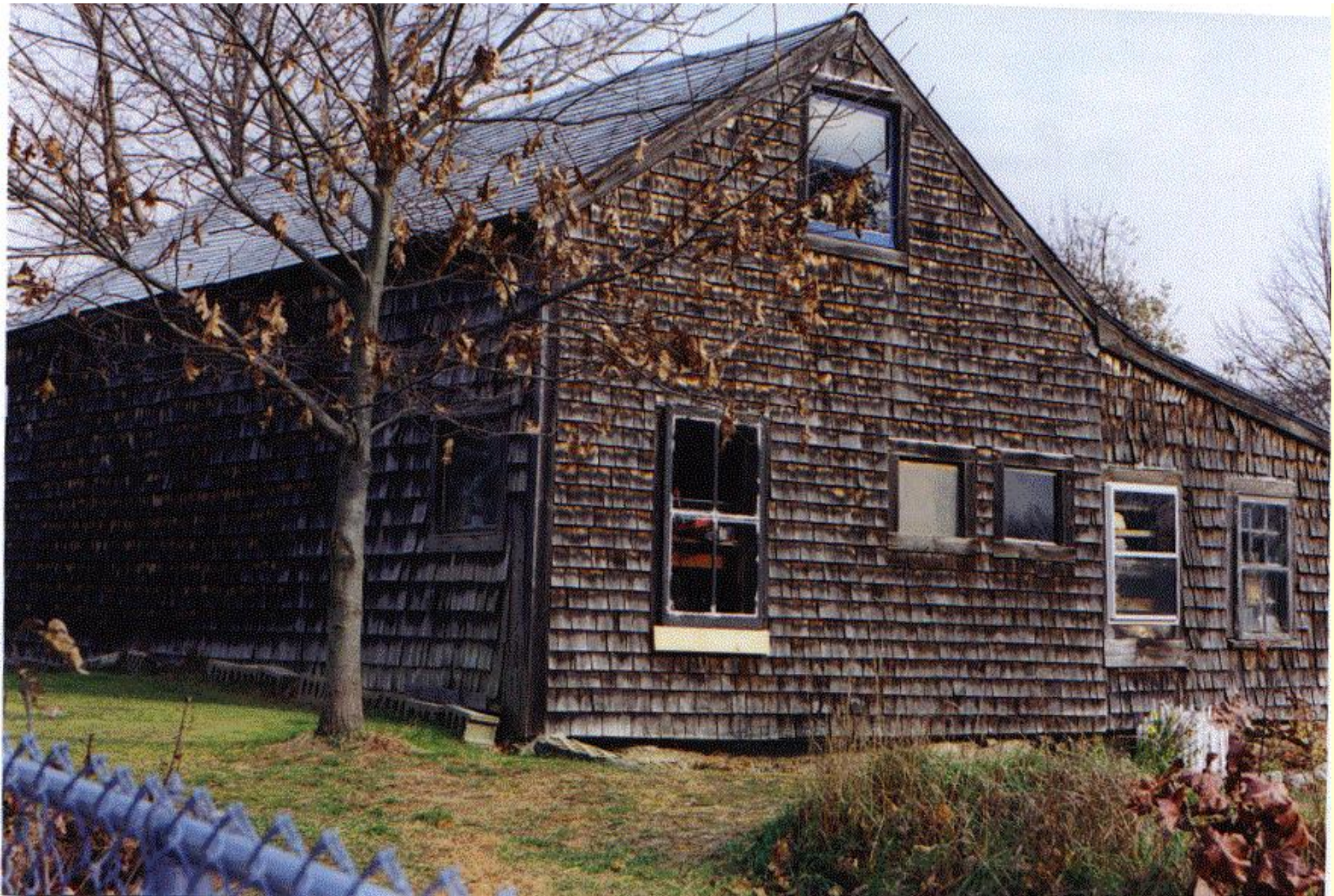
The weathered gray shingles of the shed, however, attest to age. One can imagine that at one time a barn, larger than the house structure itself, sat nearby.
